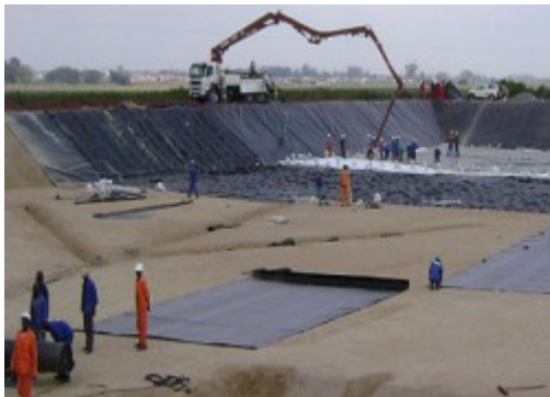
The Johannesburg Water's Olifantsvlei Wastewater Treatment Works Module-3
